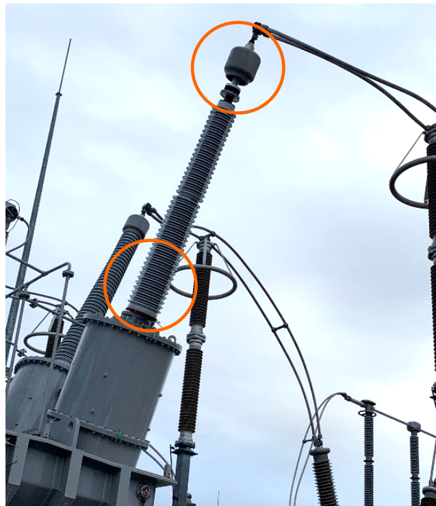
Fig. 21. Damaged reactor bushing at Romney.
