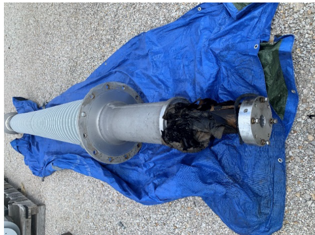
Fig. 22. Removed damaged reactor bushing at Romney.
