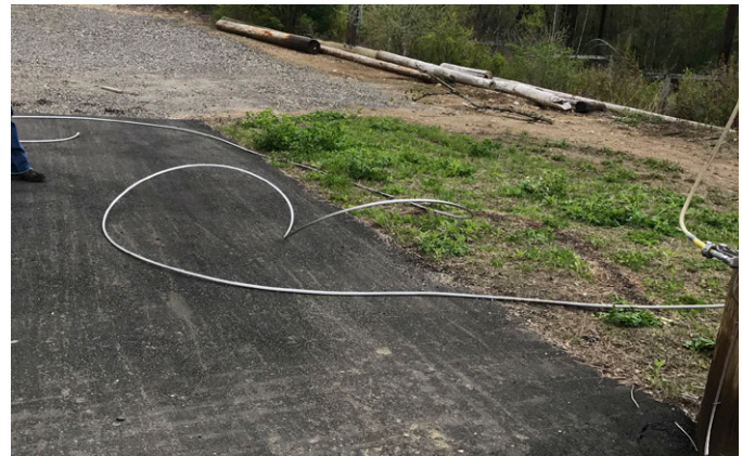
Fig. 12. HIF Test 1 with the downed conductor lying primarily on asphalt with secondary grassy contact.
