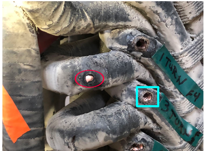
Fig. 19. Photograph showing the tapped fault point in the stator winding (blue rectangle) and the remainder of a sheared-off bolt (red oval).
