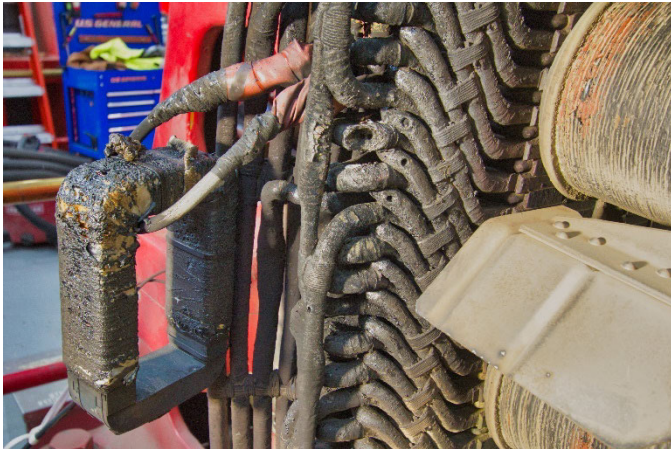
Fig. 21. Photograph showing the damage to the stator windings and one of the branch CTs after a branch fault evolved into a phase-to-phase fault.
